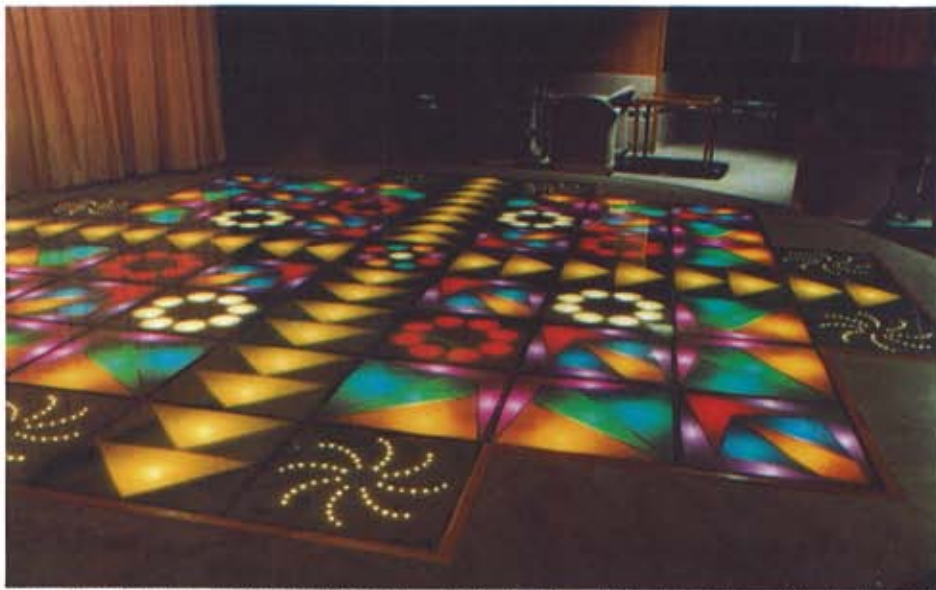
Novas manufactured and installed this Graham Fathers' designed illuminated dance floor in the Carib Lounge of the Sea Princess. There are five wiring circuits, two 4 x 4 matrix, and three 4-channel geometrically interlaced, but electrically separated, giving numerous effect options.
