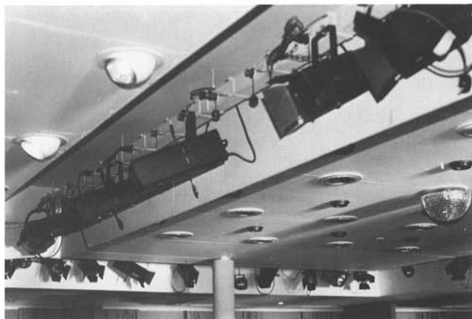
The Ocean Room in the S.S. Canberra - the low deck-head poses obvious problems for any lighting installation.
